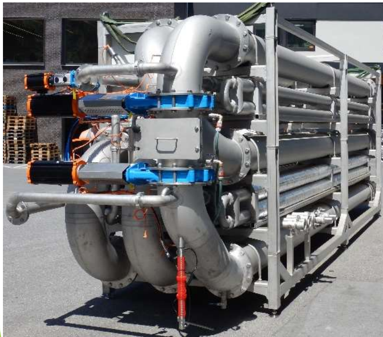
Continuous sludge pasteurisation
